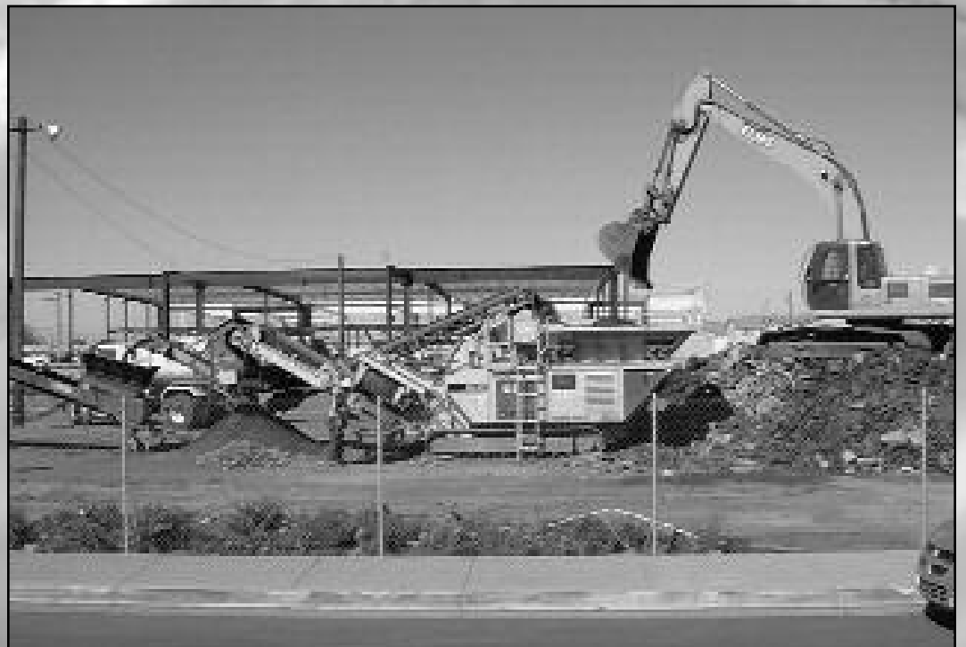
Huge machinery and piles of aggregate front the construction site of the new Rogers and Rogers Toyota building at Highway 86 and Wall Road. It follows the recent completion of the dealership's new Nissan facility.
