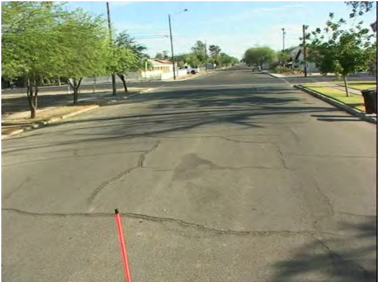
F Street, PCI = 58, The Cracking Tends Further Apart, Non-Load Related and Sealed
