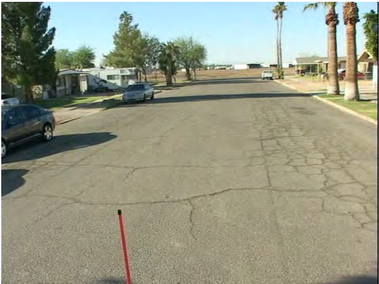
G Street, PCI = 39, Just Starting to Fail in Larger Areas and Becoming Rutted
