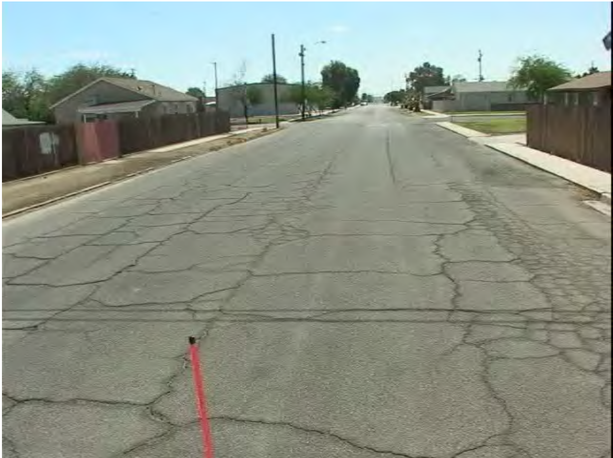
7 th Street, PCI = 33, This is the Worst Part of the Roadway
