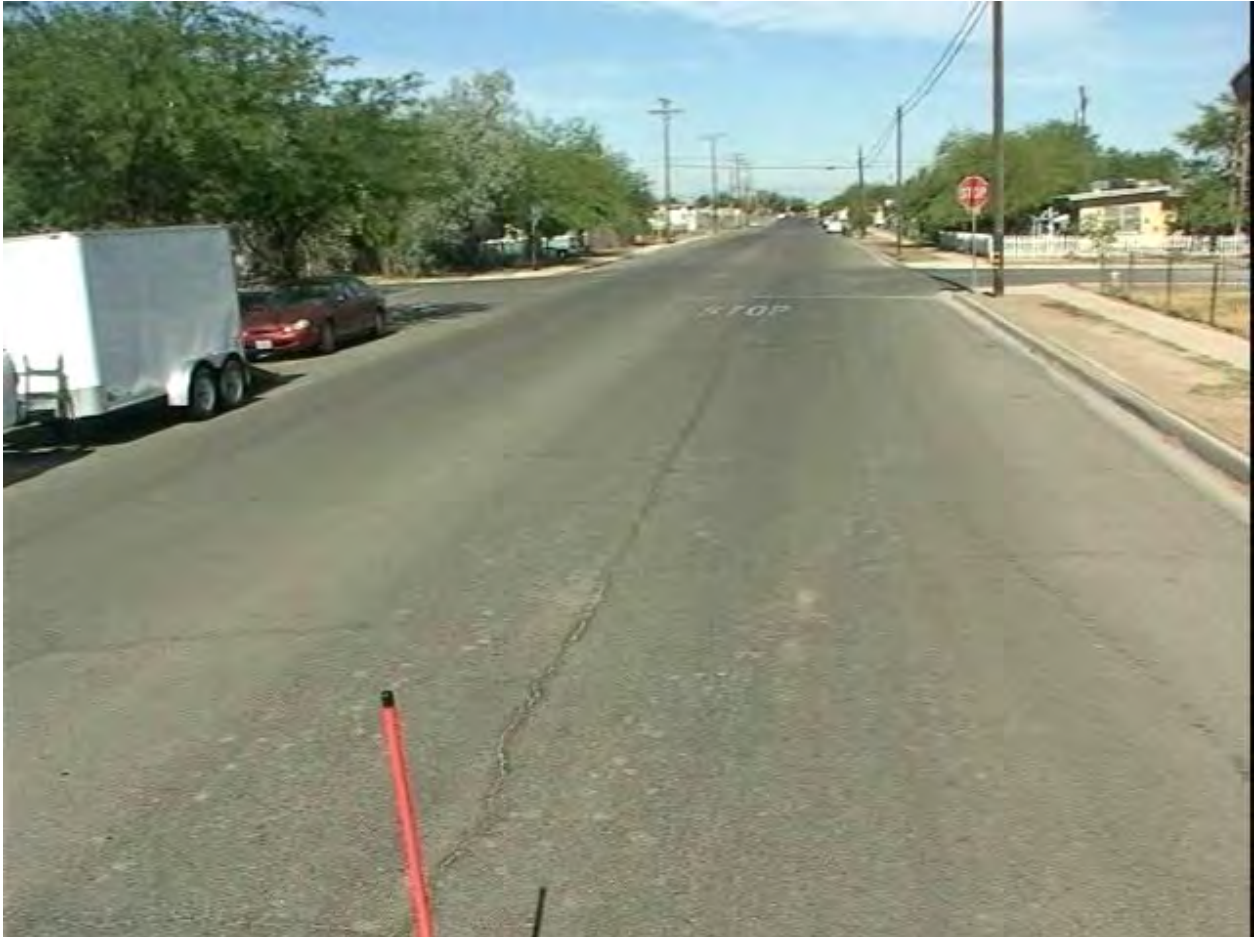
12 th Street, PCI = 76, Performing Well With Intermittent Non-Load Related Cracks
