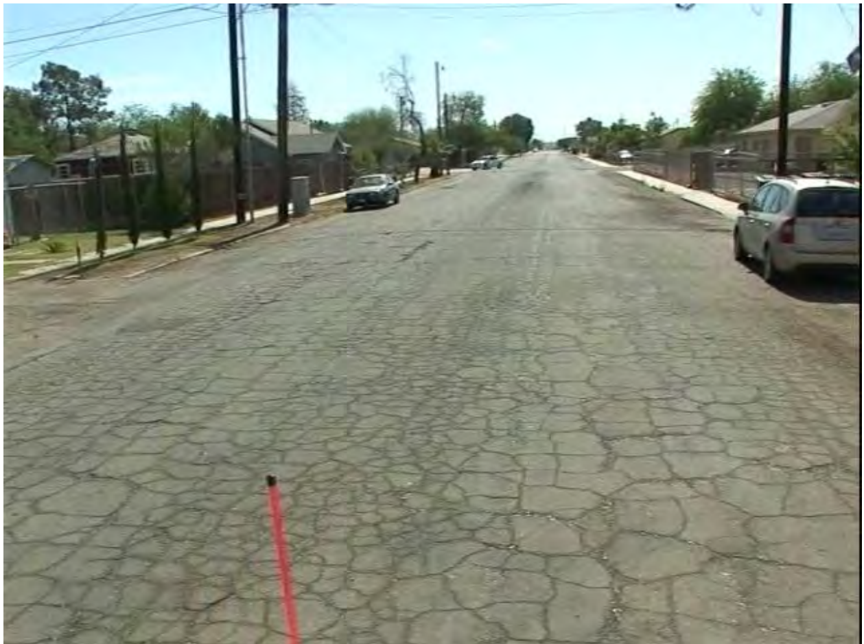
7 th Street, PCI = 19, The Entire Street Has Failed due to Poor Base Conditions
