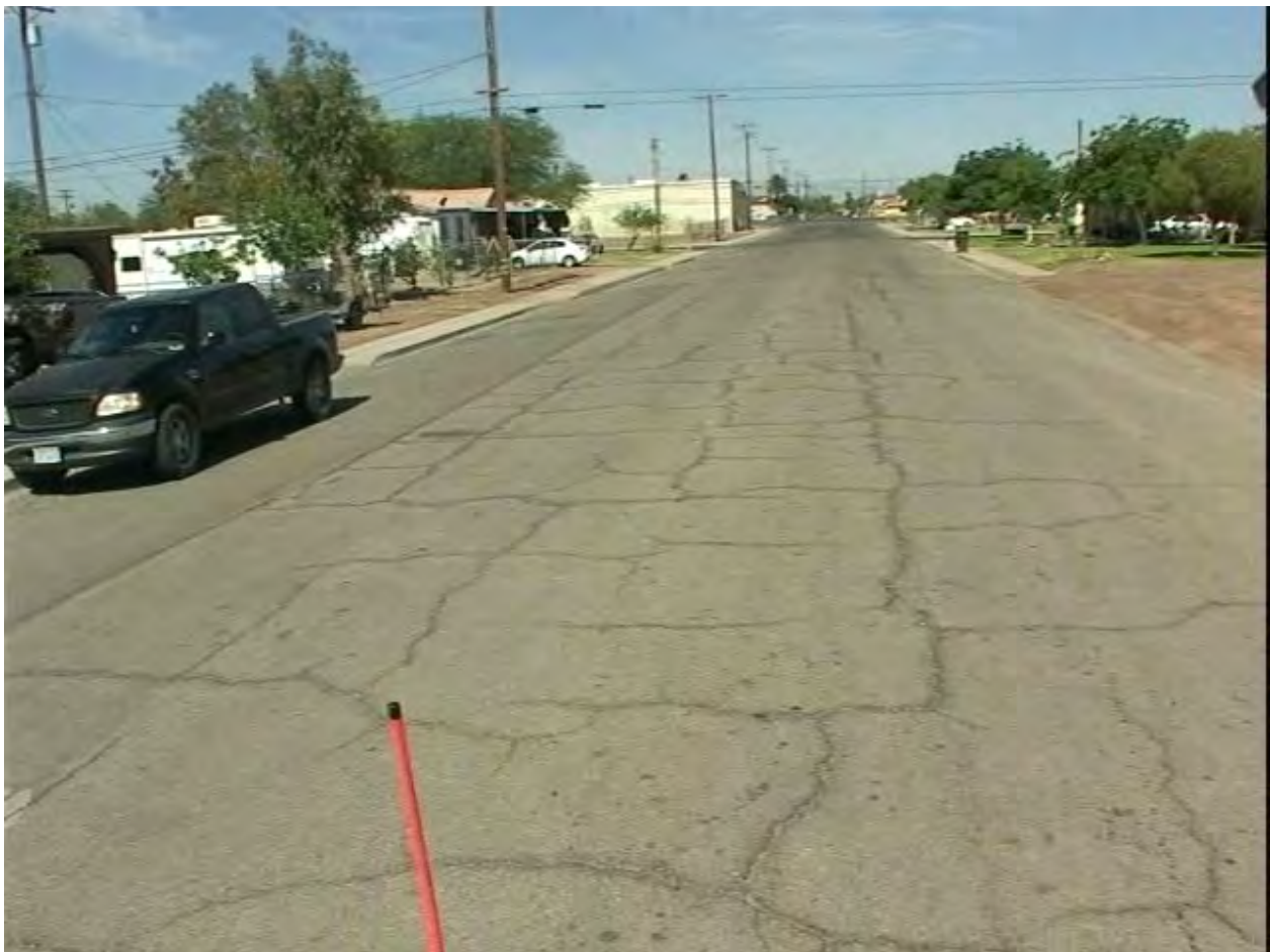
Ophir Dr, PCI = 47, Just Starting to Fail in Local Areas with Most Distresses being Non-load Related
